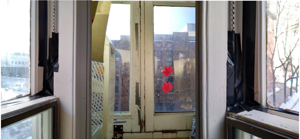
Figure 9 Examples of OSPS Windows in Poor Condition
