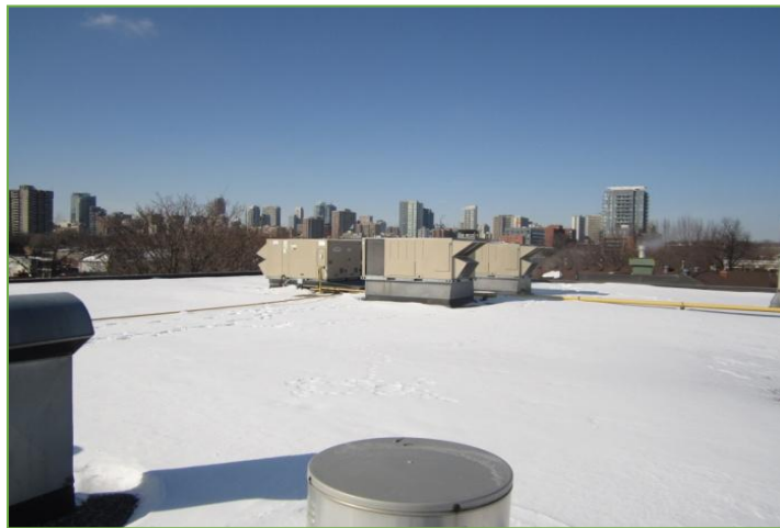
Figure 8: Rooftop HVAC Units
